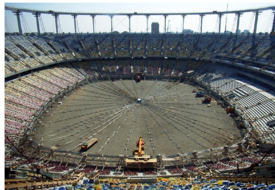
〈Fig. 8〉 The cable net structure was laid out before the lifting operation
