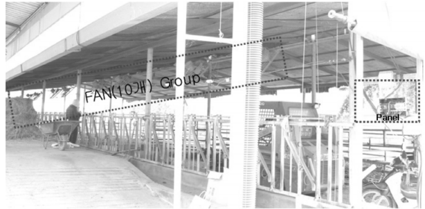
Fig. 2. Electric fan group at livestock barn.
