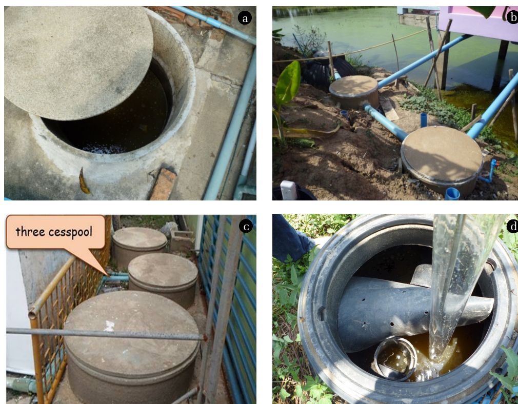
Fig. 2. Types of on-site sanitation (a) one cesspool, (b) two cesspools in series, (c) three cesspools in series, (d) commercial package.
