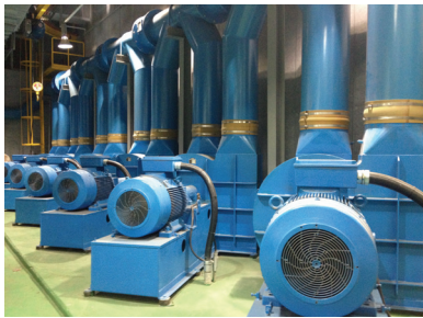
Fig. 2 Blower system installed at the domestic site of a automated vacuum waste collection system
