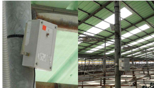
Fig. 9. Cases of test-bed installation.
