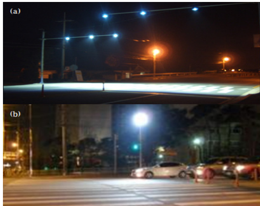
Fig. 1. Installations of LED crosswalk (a) division of LED crosswalk, (b) a single of LED crosswalk.
