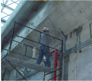
Fig. 2 Leakage at construction joints
