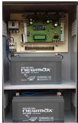
(b) Controller and battery
