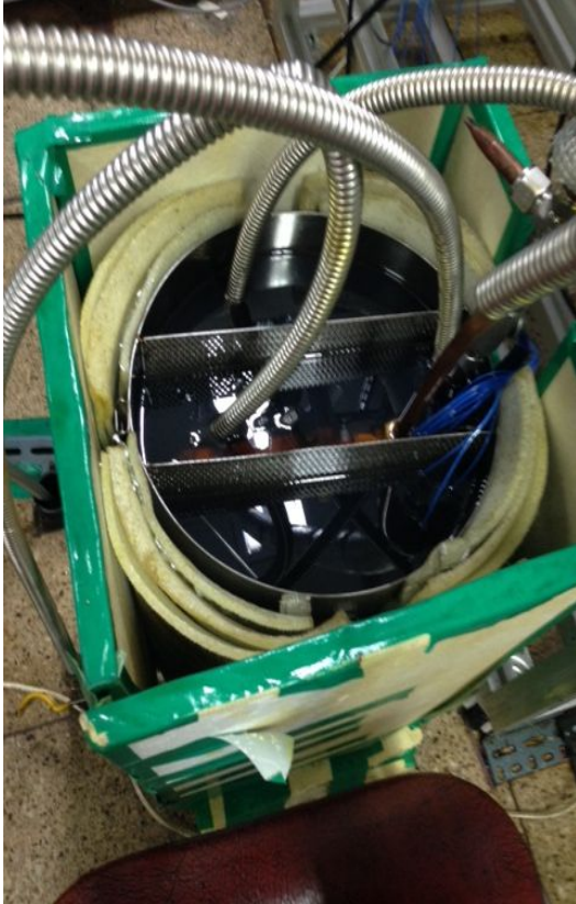
[Fig. 4] Oil tank and evaporator
