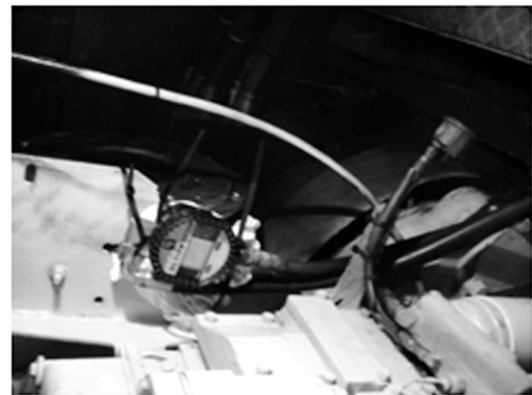
Fig. 1. The Installed flowmeter in the engine room of Haengbok-ho.
