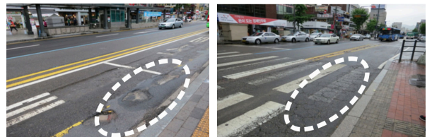
Fig. 4 Damages Near Bus Station
