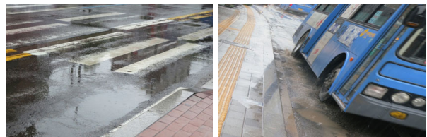
Fig. 5 Ponding Near the Bus Station the Rainy Season
