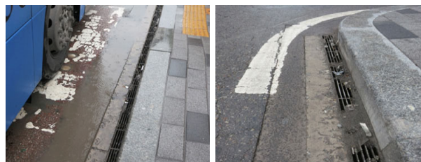
Fig. 14 Bus Stop Drainage
