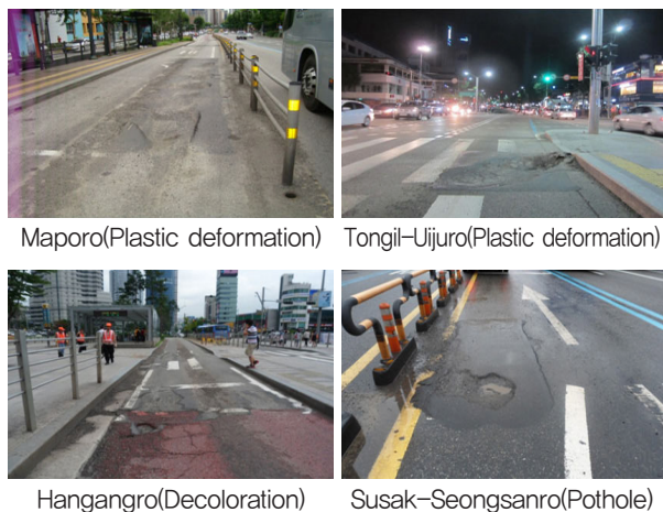
Fig. 3 Bus Rapid Transit Pavement Damages
