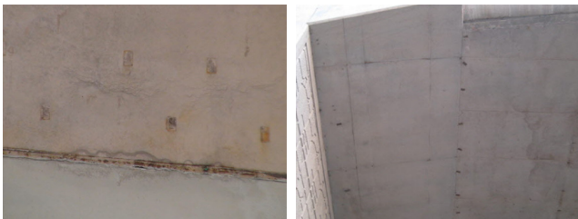
(a) Cracks around spacer (b) Crack free around spacer
