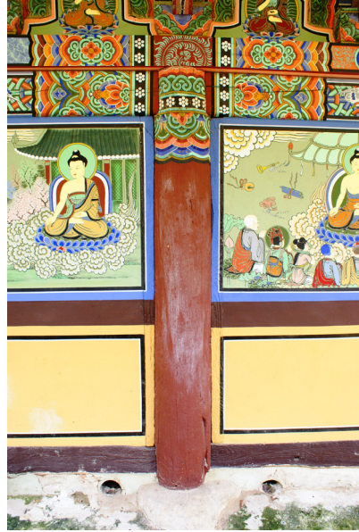
Fig. 2. Efflorescence damage after FRT (Gyeonggi Anseong Seoknam-sa temple).
