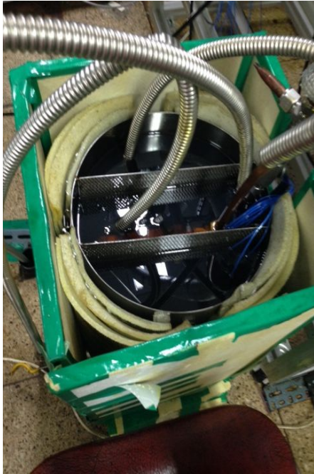
[Fig. 4] Oil tank and evaporator
