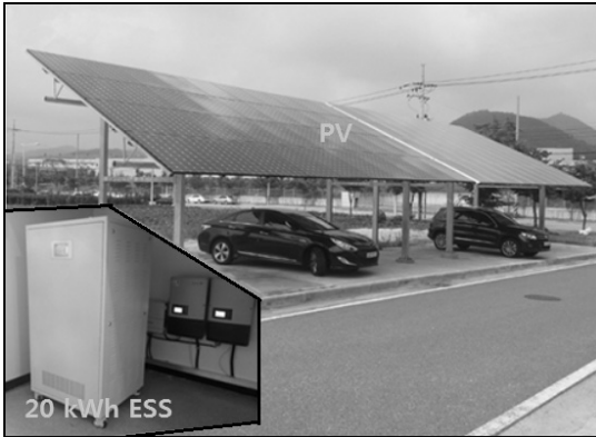
Fig. 2 ESS and PV installed at Hydrogen Fuel Cell Center in Woosuk university
