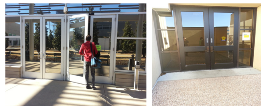
Figure 4. The entry door at most buildings has wide enough, but do not provide braille signage(UTD).
