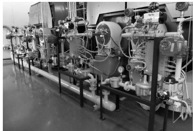
Fig. 1. City gas boiler(indoor)
