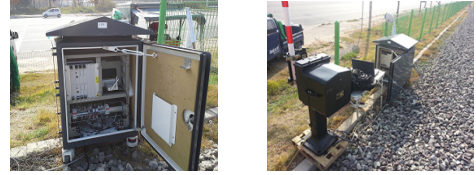
(a) WOCU for crossing gate (b) Crossing gate
