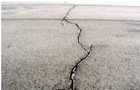
(b) Crack Propagation Shape
