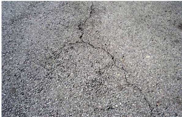
(a) Initial Crack Shape
