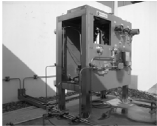
Fig. 3. HCNG mixing equipment.
