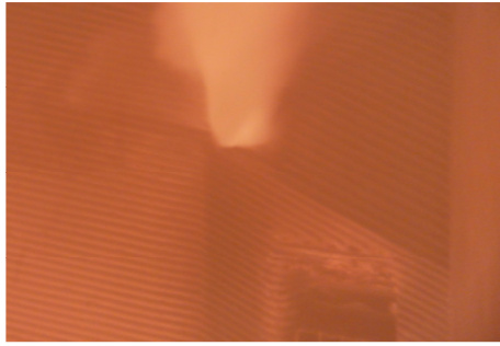
Fig. 1. Boiler waterwall tube rupture of T-Powerplant
