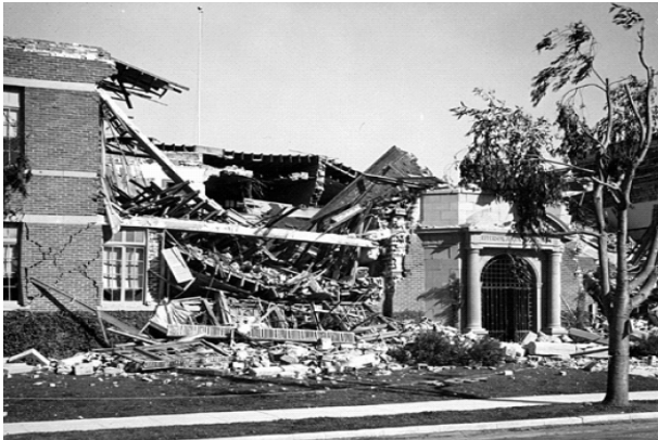
Figure 1. Earthquake damage of school building in CA, USA
