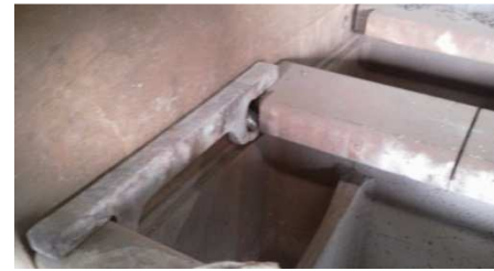
(b) Great-Bar corrosion
