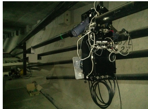
Fig. 15 Field test for integrated cable NDT system
