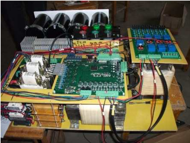
Fig. 21. Implemented LCL filter-based shunt APF system.
