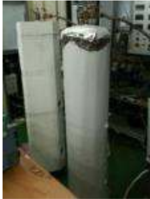
Fig. 5 Type 1 CMI and EPS installation heat storage tank
