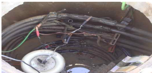
(b) First joint measured surge overvoltage
