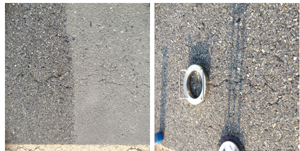
(a) Sections of Treatment(left) and Untreatment(right) with HL-TM (b) Preparation on the Crack Section
