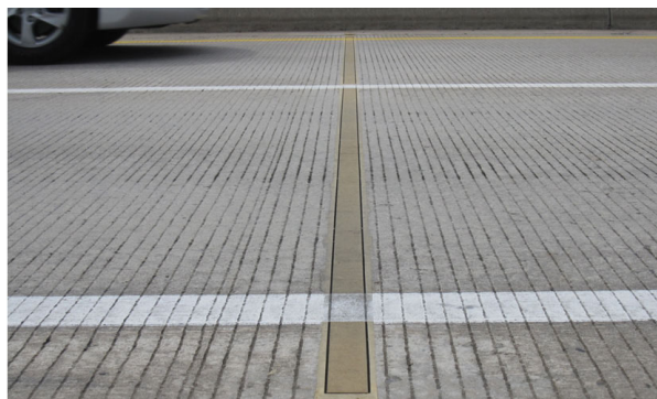
(b) Installed WIM Sensor (Piezo-Quartz Type)
