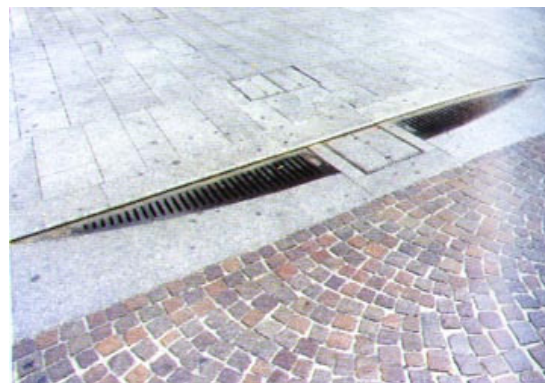
Fig. 2. Willow-Shaped Rainwater Well Cover.
