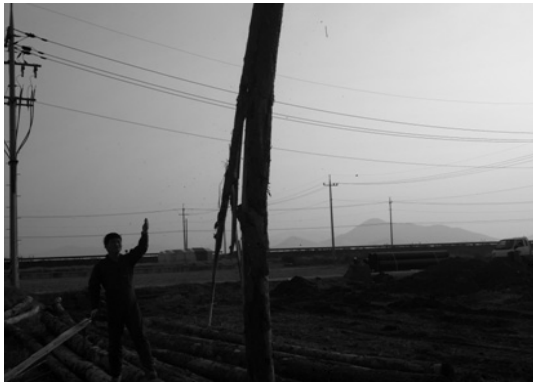
Fig. 6. Breaking of wood pile.
