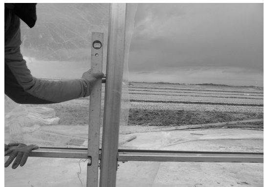
Fig. 9. Tilting of column.
