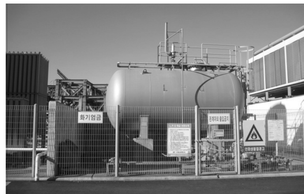
Fig. 1. LPG storage tank.
