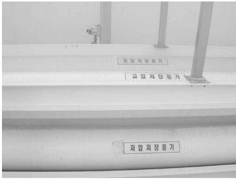
[Figure 2] Hydrogen gas storage vessel
