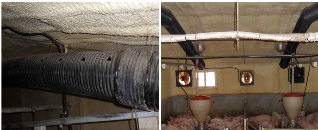
Fig. 1. Circular duct and exhaust fan of ventilation systems at swine facility.
