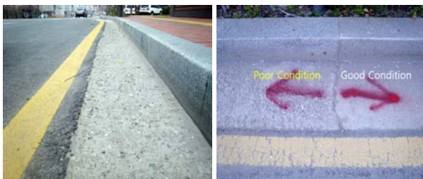
Fig. 4 Picture of Scaling Failure
