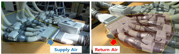
Fig 5. Air distributor of supply and return line
