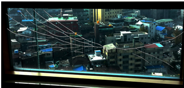
Fig 2. glazing breakage due to thermal expansion
