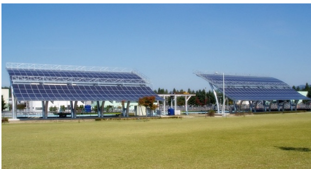
Fig 2 Photovoltaic system of C city sewage treatment plant
