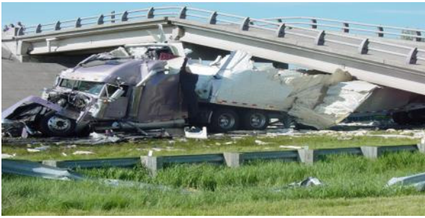
Fig. 1 Bridge collapse due to a truck collision(NDOR)
