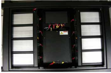
Fig. 7. Lithium polymer battery pack (250V/10Ah).
