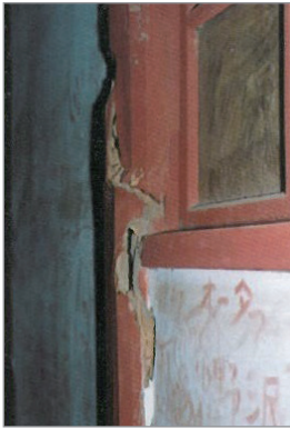
Fig. 2. Temple damaged by termite.
