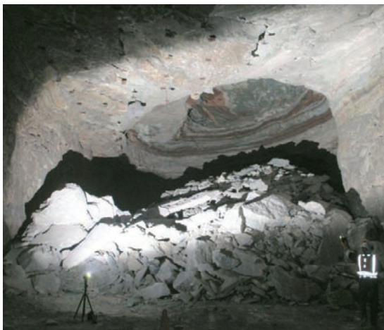
(a) Roof failure
