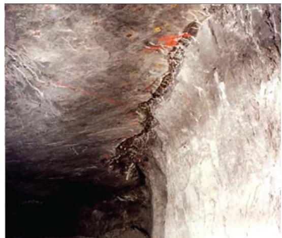
(b) Failure at the pillar-roof contact
