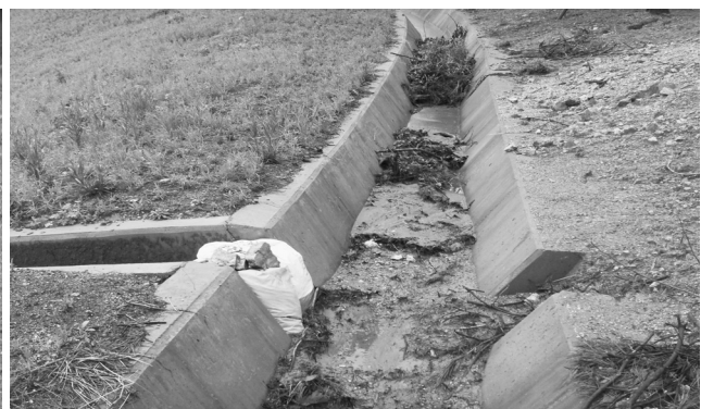
(b) Loss of Gutter Ability by Debris
