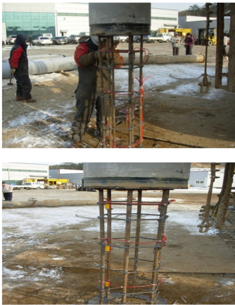
(a) Steel Connections
