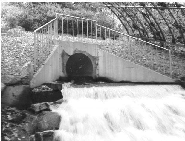
Fig. 2. Effluent discharge outlet of Kiheung Respia treatment plant for the micro-hydropower installation.
