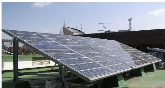
Fig. 3 3kW grid-connected PV system
