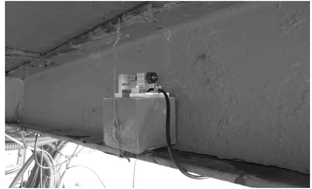
Fig. 5. Crackmeter installed in marine biology laboratory
