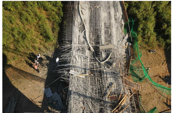
(b) Top view of the accident scene
