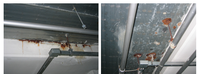
Photo 1 Rust of steel wire integrated deck plate system
