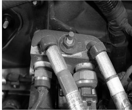
Fig. 3. LP gas connecting hose of normal state.
